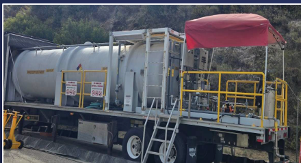
Mobile hypochlorite tanker and pumps
