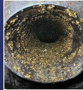
Pipeline (photo: Arvin Edison Water Storage District)
