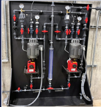
Chemical pump skid
