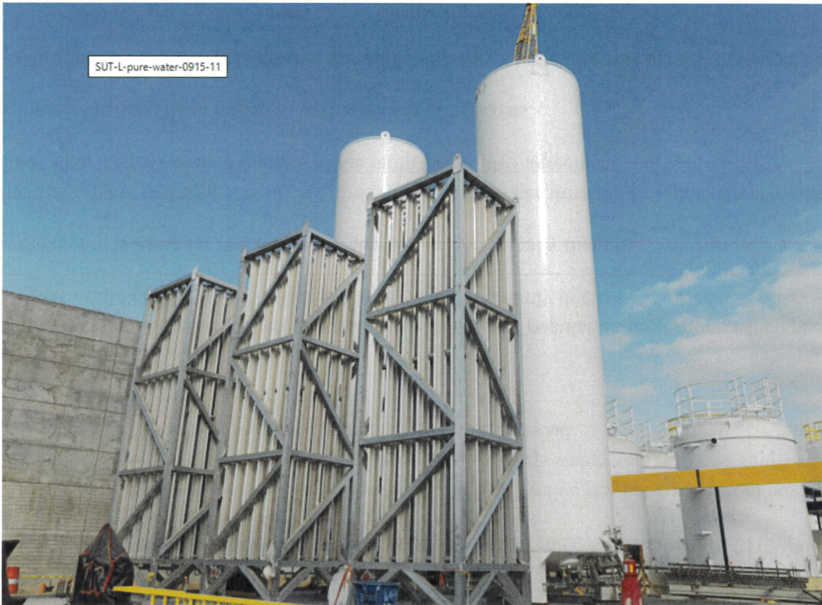
Liquid oxygen tanks at the Pure Water facility under construction in San Diego two years ago. (Ana Ramirez / The San Diego Union-Tribune)
