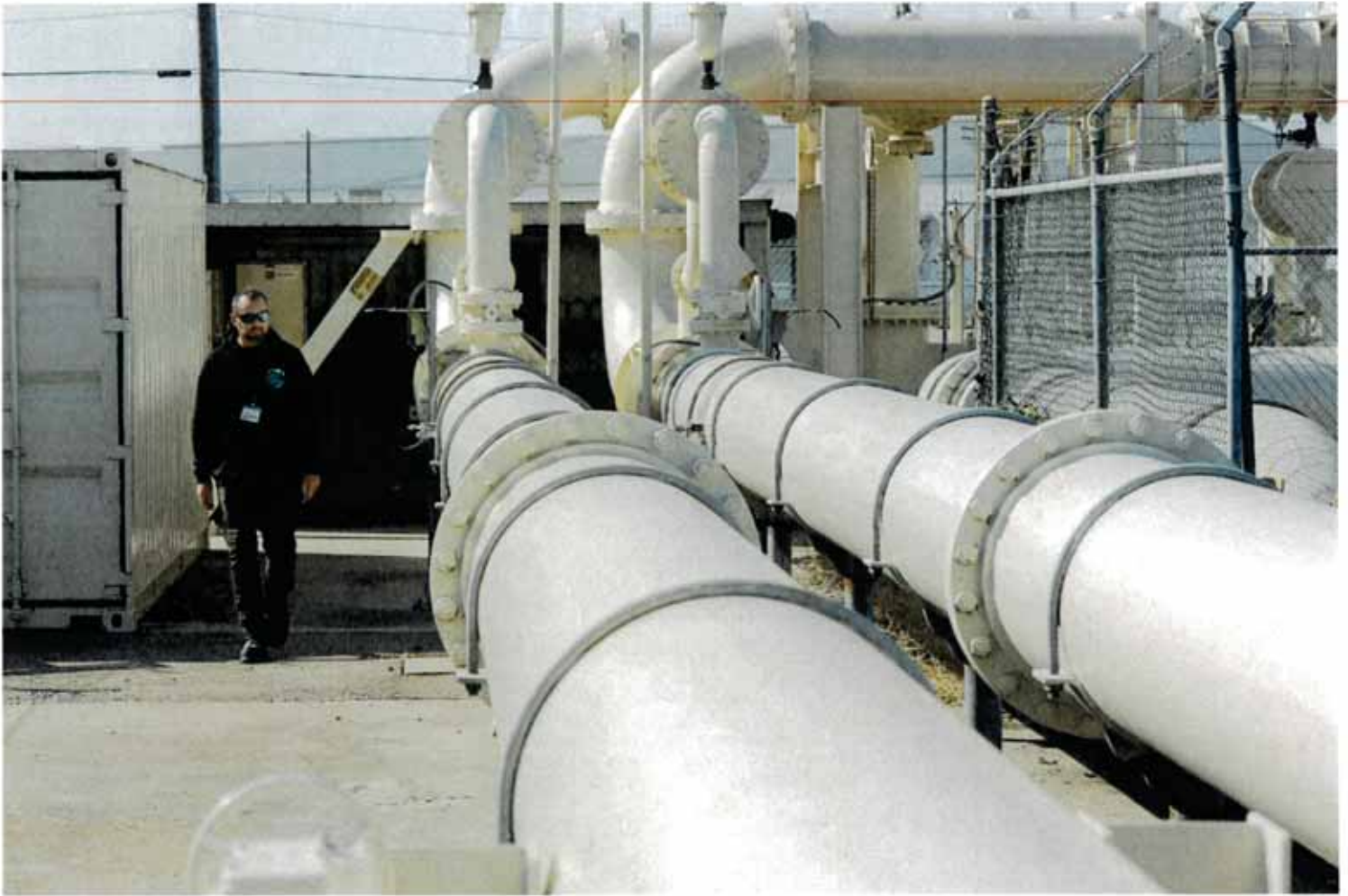
Port of Stockton employee Steven Bender inspects equipment used to aerate water at the Port of Stockton on Oct. 23, 2025. Golden mussels spread rapidly and can damage pipes and pumping equipment, leading to costly repairs. Photo by Fred Greaves for CalMatters
